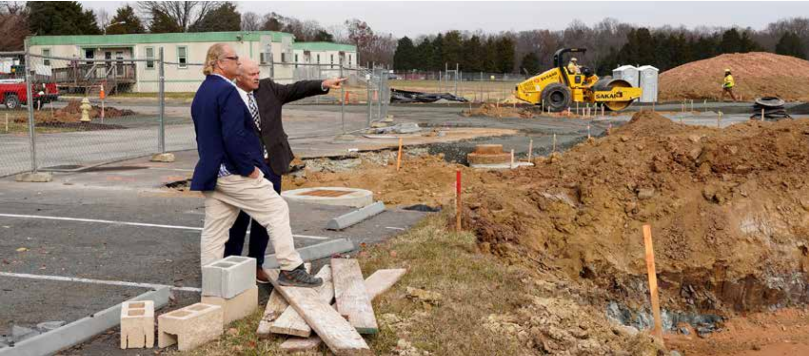
YFT Trustee Danny Hazel, son of the late YFT benefactor William A. Hazel and YFT Chief Financial Officer & VP of Operations, Rich von Gersdorff inspecting the site preparation work by the William A. Hazel Co. crew.
